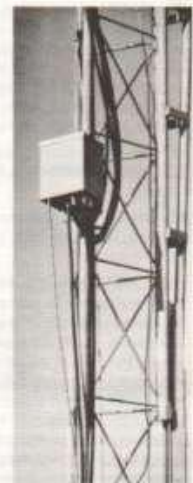
Remote Switch installed on tower
