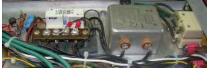
Figure 1.8 Inrush Current Limiter & RF Line Filter Installation Original AC Circuit breakers on right hand side
