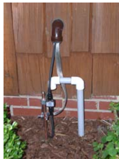
Shack end - Ground Rod and PolyPhaser protection
