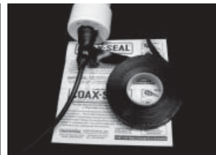
Optional, but recommended, apply a layer of Cold-shrink tape completely over the Coax Seal.
