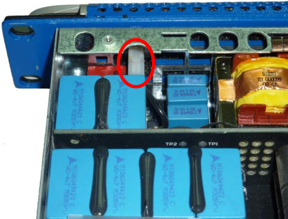
Amplifier power switch cable to be disconnected
