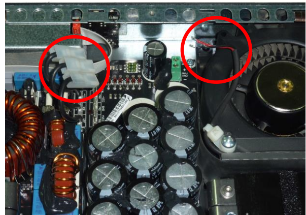
Disconnected fastons between power supply board, output amplifier board and fan power cables
