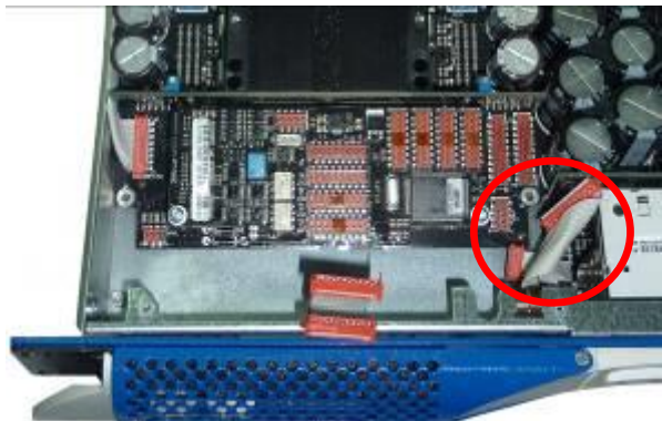
Control board flat cables unplugged
