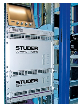
Floor specific equipment room with SCore
