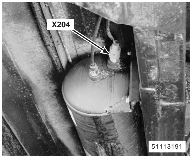
193. beneath LH side of vehicle X204 Reservoir Pressure Switch
