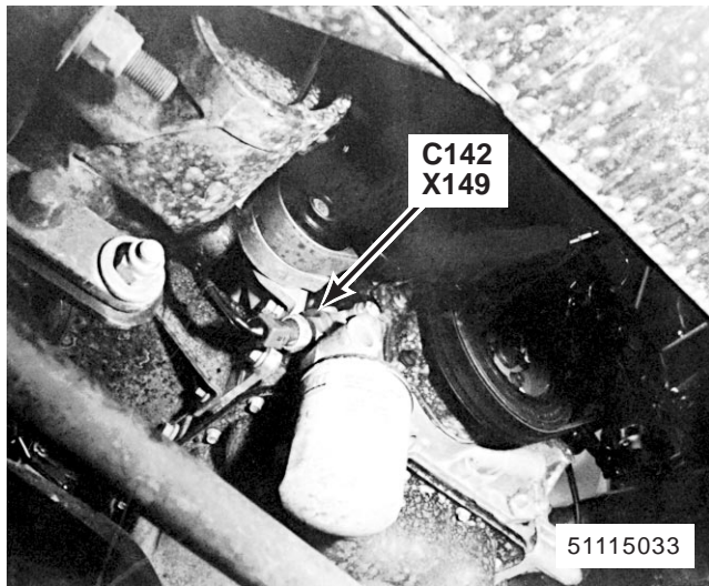
35. lower RH side of engine MFI-T16 X149 Oil Pressure Switch C142 (2-N)
