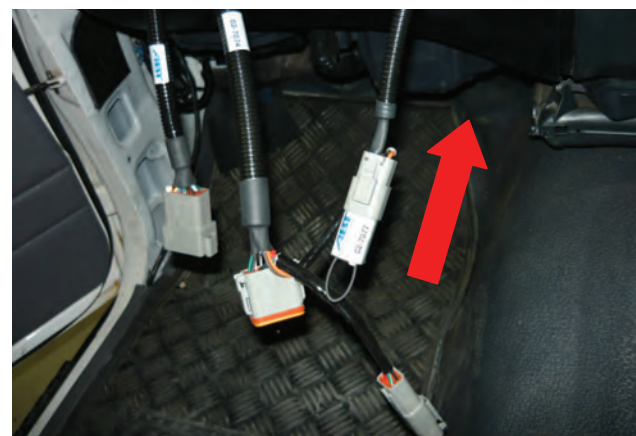
Figure 67: Cabin control harness fed into glove box
