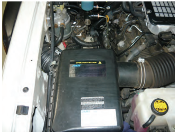
Figure 121: “Operator Caution” label under bonnet.
