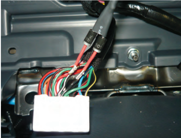
Figure 85: Solder splice into the Black and Black/ White multi-plug cables.
