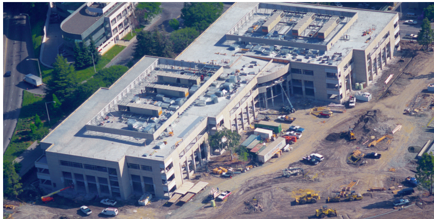
Agilent Technologies new headquarters rises on the same site in Palo Alto where Dave Packard and Bill Hewlett built their first factory, The Redwood Building, in 1942.
